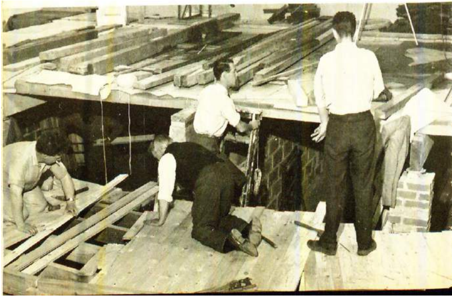
Figure 1. Bristol Arts Centre auditorium under construction, c. 1964. BFI, The BFI in the Eighties: The work of the British Film Institute and its plans for the future: a report produced on the occasion of its 50th anniversary in 1983 (London: BFI, 1983), 22.
